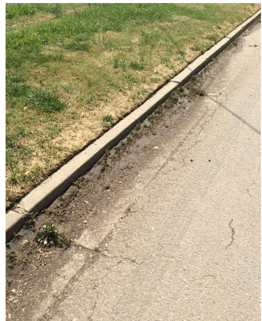
Figure 21. Sediment laden gutter pans along Slagle Avenue.
