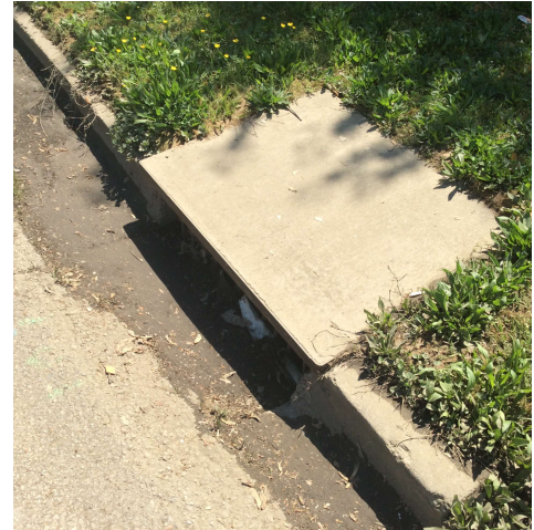
Figure 16. Sediment in the gutter pan along Slagle Avenue.
