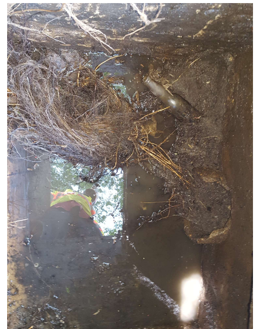
Figure 9. Even after cleaning the inlet, trash, root masses, and sediment clogging the storm drain system remain. The City's infrastructure is old, inadequate, and ineffective.
