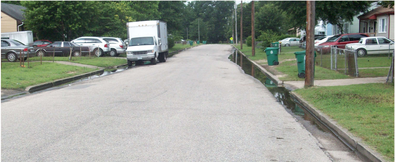
Figure 18. Stormwater extends from inlet to inlet across N. Whitehill Drive during precipitation events due to lack of adequate drainage infrastructure.
