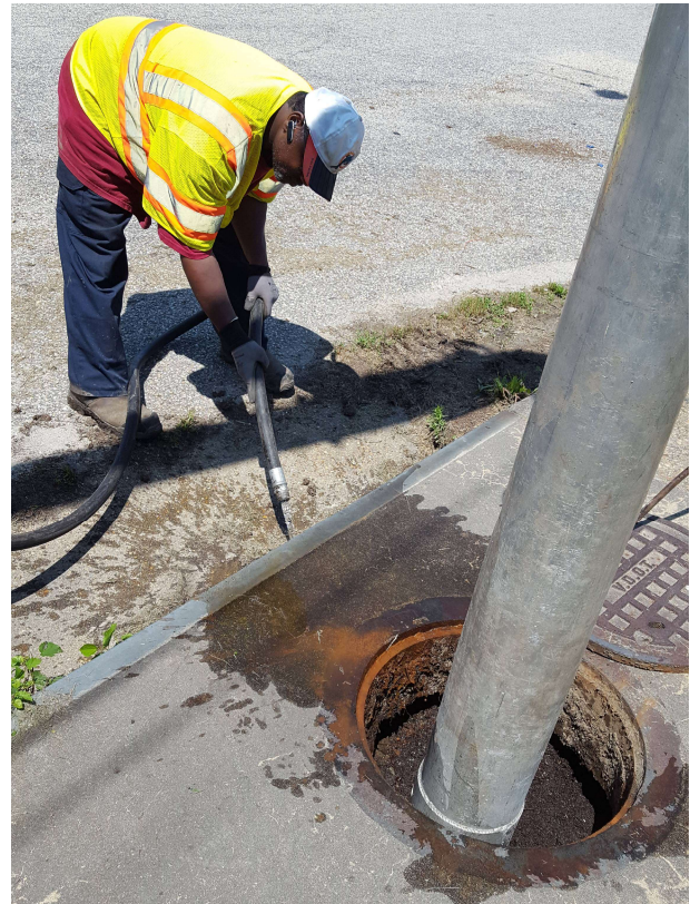
Figure 26. Jetting and vacuuming the inlet filled with sediment at the intersection of Courthouse Road and Richmond Road.
