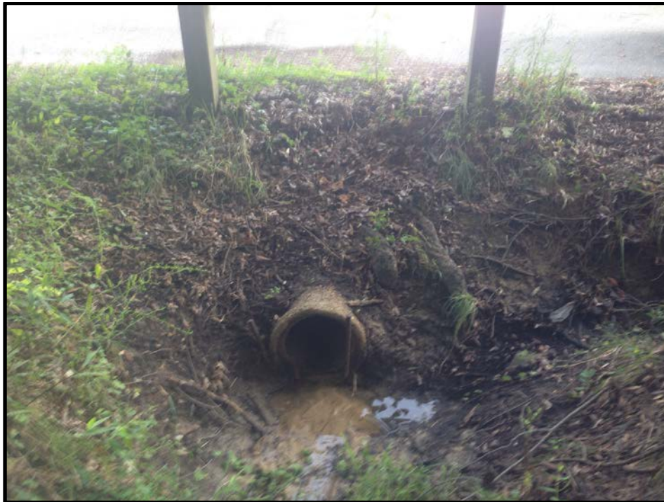
Photograph 4 (P4) – 12 inch RCP which serves as the only visible outlet for the 85.52 acre watershed system draining to this point. View is northwest August 2017 – P. Sharpe.
