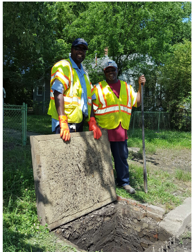
Figure 7. City Streets Operations staff assisting with drainage investigations by jetting and vacuuming inlets and providing access to the drainage team on May 24, 2018.
